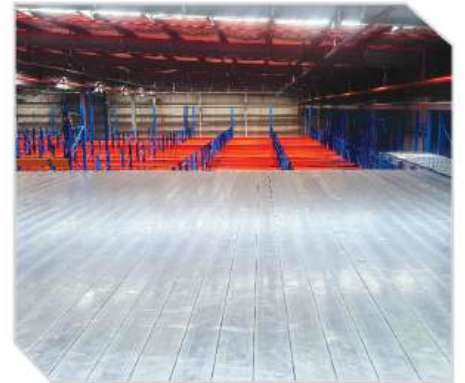
Rack Supported Mezzanine floor
