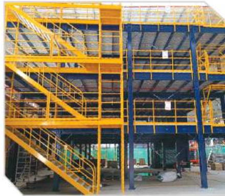
Multi Tire Mezzanine floor
